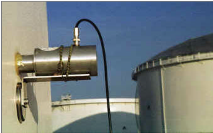
Sonar Transducer Listens Through a Tank Wall
